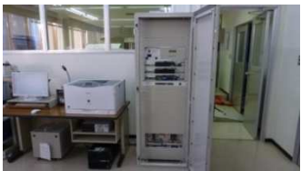
Dam Observation Data Management Equipment in the Central Control Office
