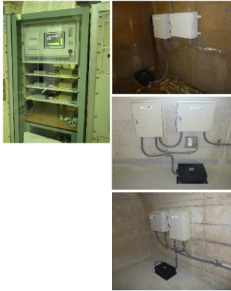
Data Processing Equipment (left) and Seismic Intensity Meter (right) from the Upper, Grout Tunnel, Top of Dam and Base of Dam
