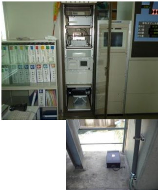
Seismic Intensity Observation Systems (upper) and Detector (lower) at Heisei Ozeki Dam
