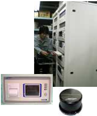
Server System at the Prefectural Office and Seismic Intensity Meter (below)
